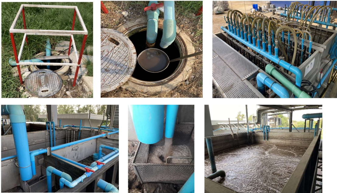
Waste water treatment system
