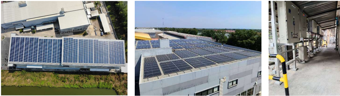
Solar power generation system (Solar Rooftop) on the roof of the factory buildings
